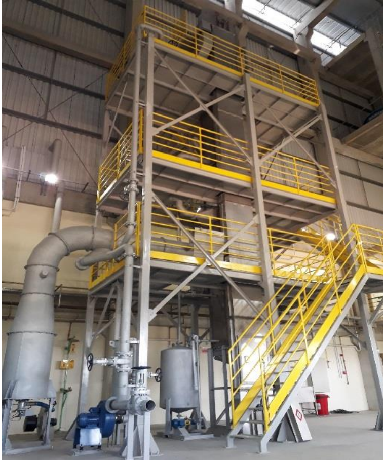
Front view of the pilot plant without thermal insulation.
