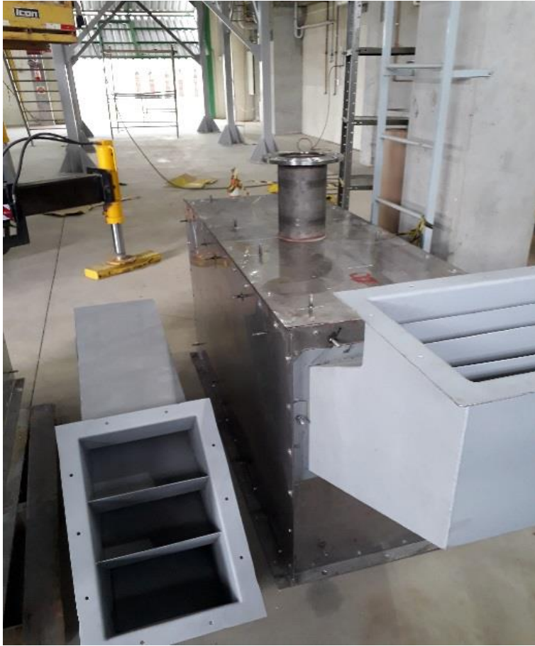
Top of the column, zeolite recirculation section for distribution in the adsorption section.
