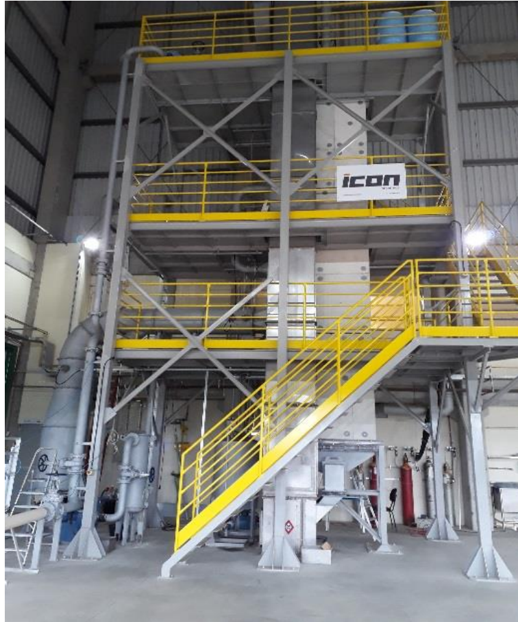
Front view of the pilot plant with thermal insulation.
