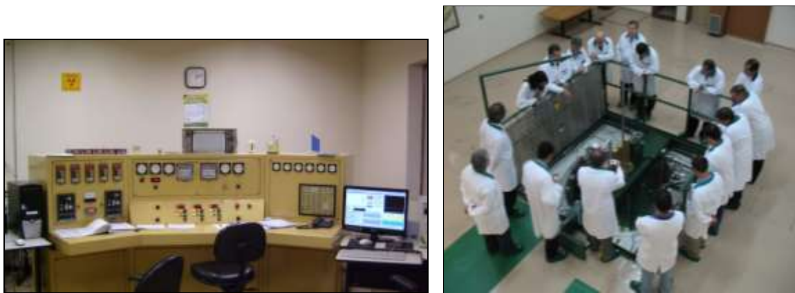
Figure A.2 - IPR-R1 – Control Room and NPP Operator Training Course
