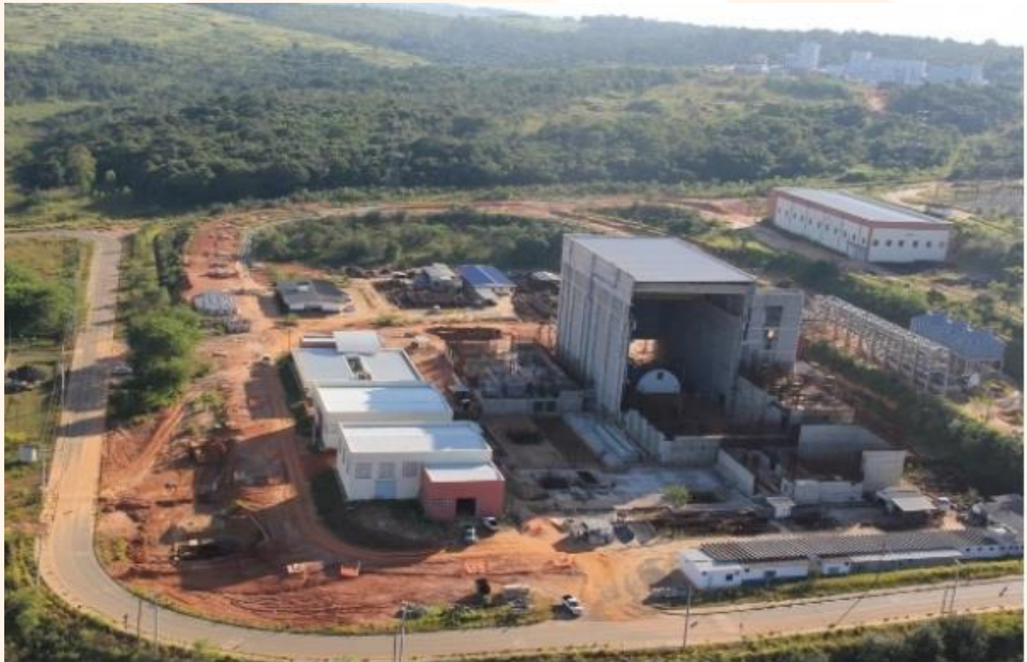
The Laboratory of Nuclear Electrical Generation (LABGENE) Iperó/SP
