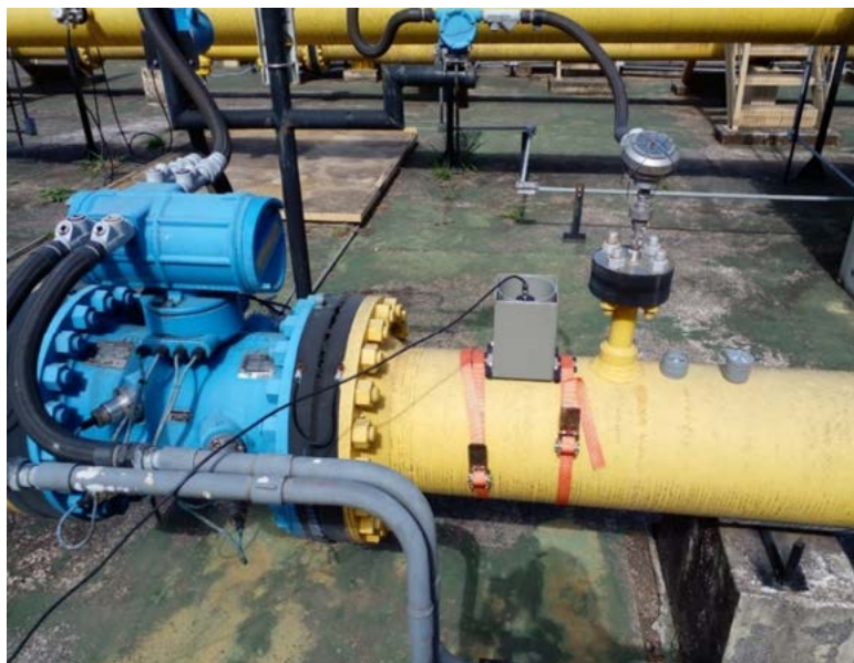
(Photo: Collimator/scintillator detector set fixing device in a natural gas high pressure line. Source: IEN/CNEN)
