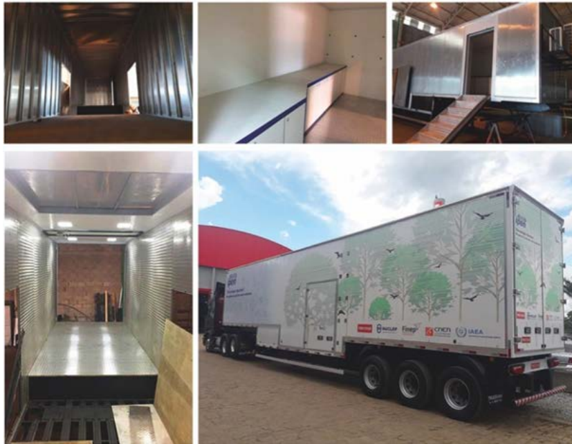
(Photos: Construction of the IPEN/CNEN's mobile electron beam irradiation unit. First photo in second line shows the radiological shielding built and installed by NUCLEP in the mobile unit. Source: IPEN/CNEN)
