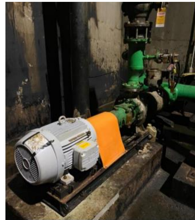
BDA-A instalada no local.
