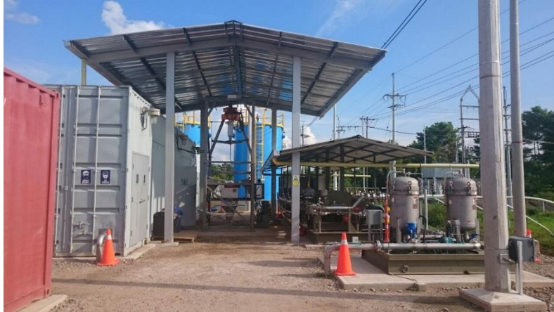
Polymer Mixing and Injection Unit
