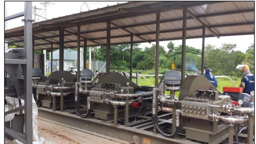
Polymer Mixing and Injection Unit
